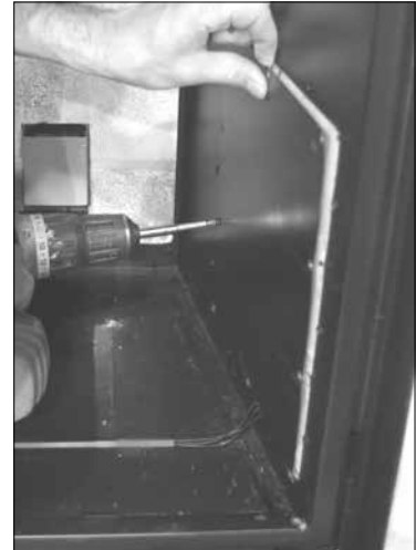
Figure 57: Removing Access Cover.
