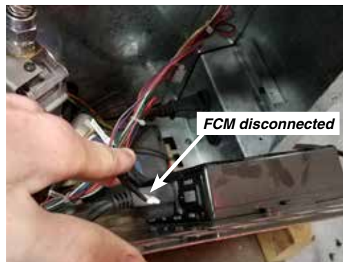
Figure 14b: FCM Disconnected
